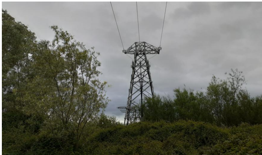
Figure 3-61: Overhead ESB utilities
